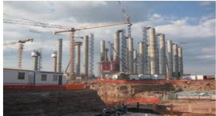
Medupi Power Station
